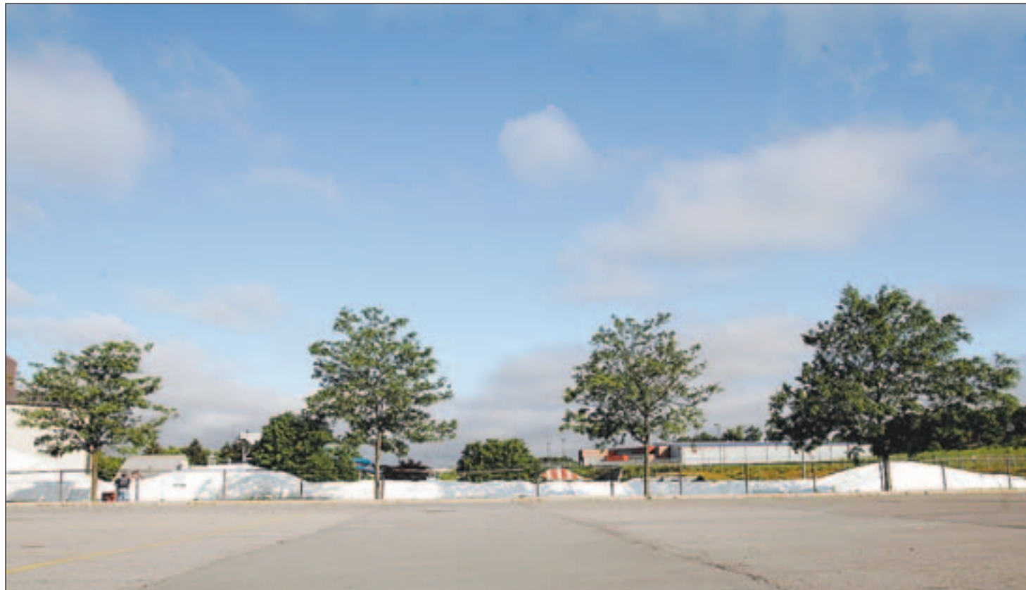
The golf dome at Sportsworld in Kitchener deflates yesterday as the new owner, GPM Managed Investments of Toronto, makes room for its redevelopment of the property with a focus on retail and office uses. It will take a few more days to completely remove the dome. Max's Golf Centre, north of Waterloo, plans to erect the dome this fall in time for the winter season. See additional photo, story on F4.
